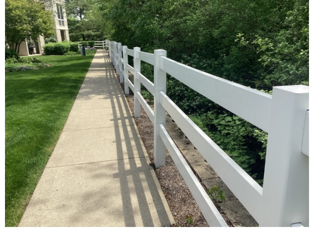
Fence leaning section
