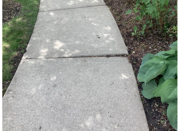
Sidewalk trip hazard
