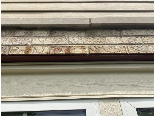
Slight lintel rust
