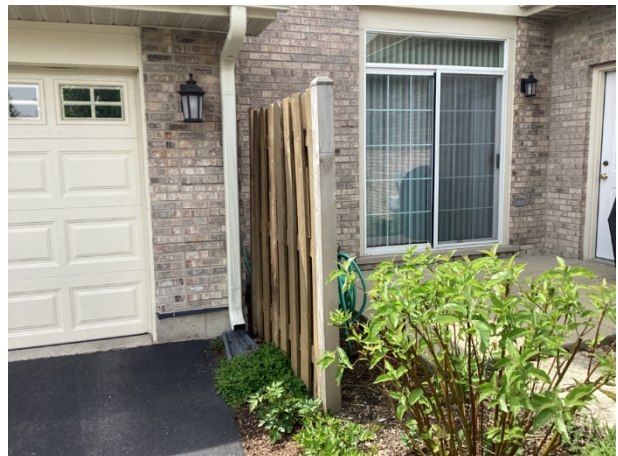
Privacy fence lean
