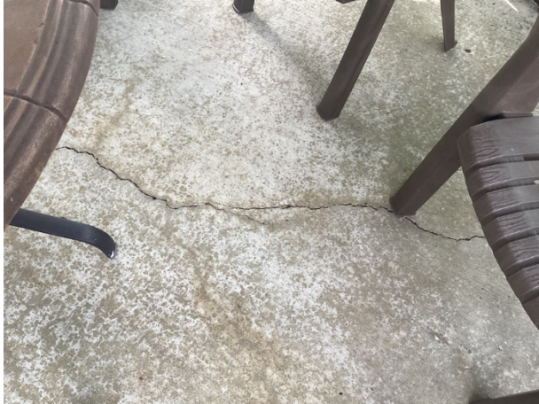
Concrete deck cracks
