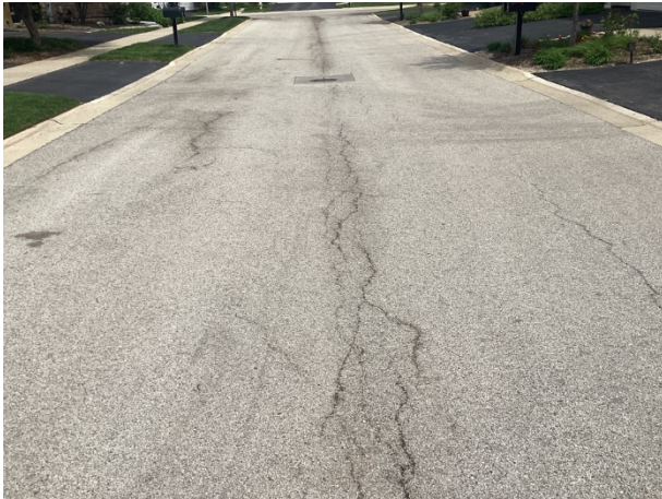
Street centerline cracks
