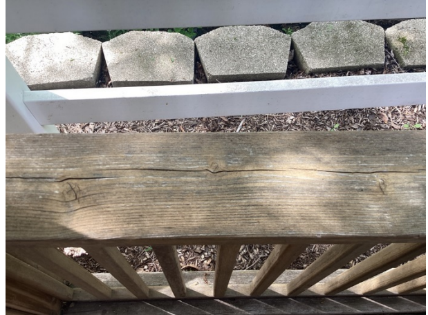
Railing wood split
