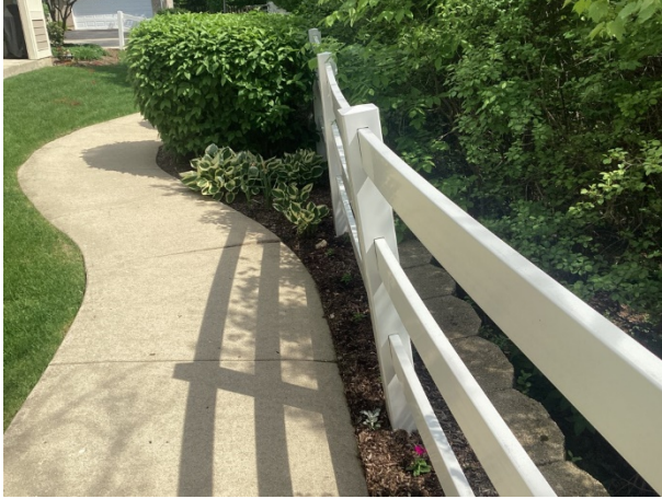
Fence leaning section
