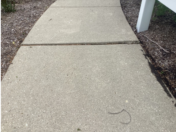
Sidewalk trip hazard
