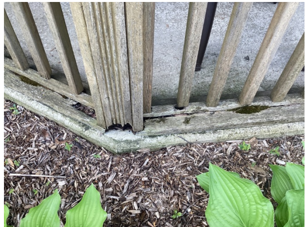
Wood rot and damage
