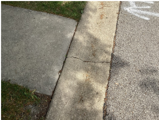
Curb and gutter crack
