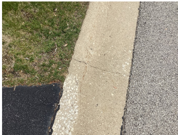
Curb and gutter crack
