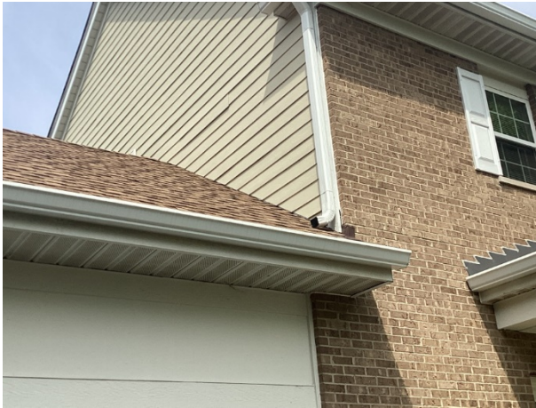
Downspout discharges directly to roof
