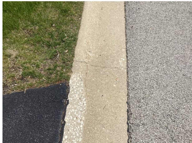
Curb and gutter crack
