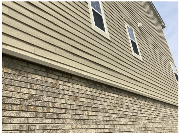
Siding deflection (640 Belmont shown)
