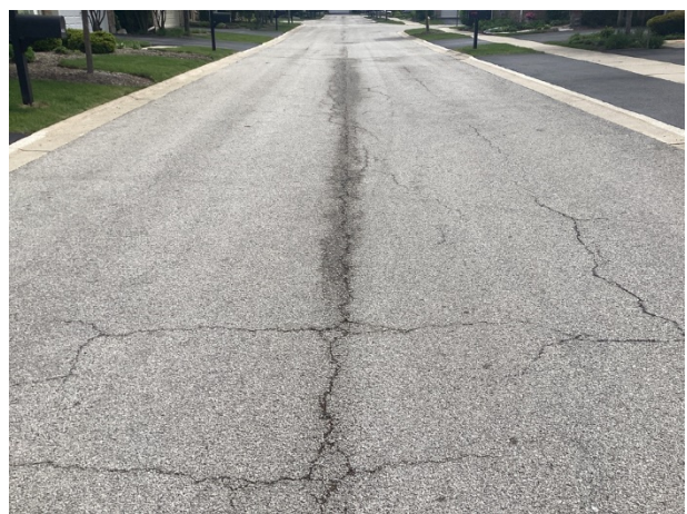
Street overview – note centerline cracks
