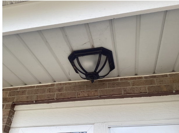
Front entry light fixture
