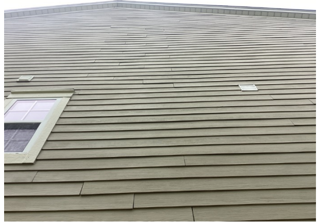
Siding deflection (479 Norwich shown)
