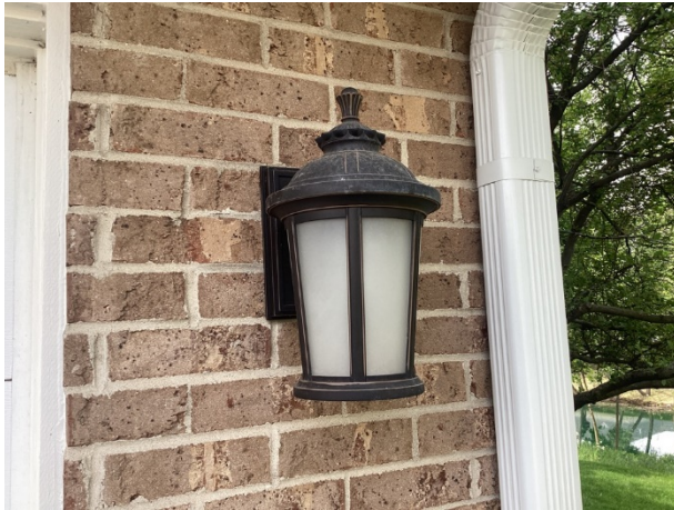
Garage light fixture
